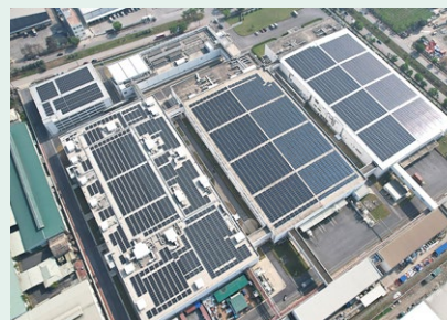
Solar power panels installed in fiscal 2022
