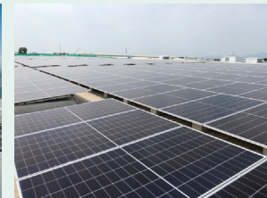
Electricity generation has begun, increasing in stages starting from August 2022
