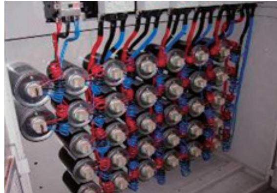
Capacitor banks to reduce phase current
