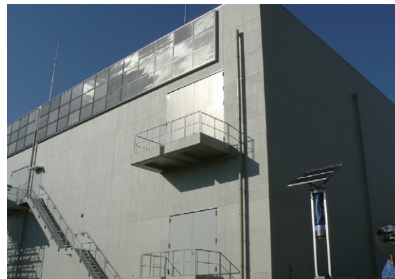
Solar panels installed at the new production building
