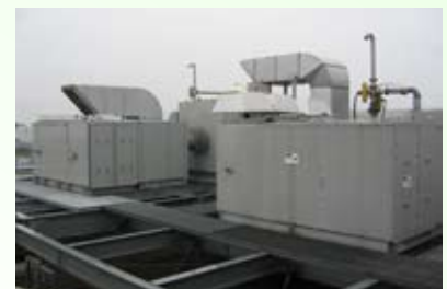
Catalytic oxidation treatment system
