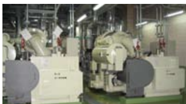
Turbo refrigeration system
