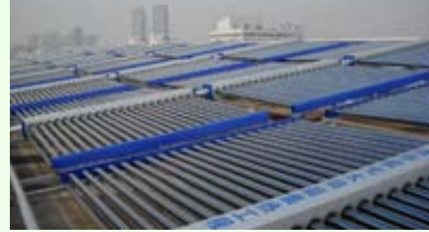
Roof-top solar water heaters
