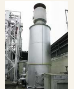
Kofu factory: Combustion chamber
