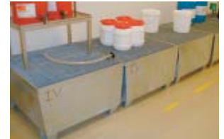
Chemical substance management The platforms on which these containers are placed have mesh tops that prevent the spread of contamination even if the chemicals leak.
