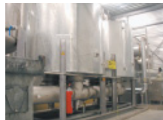
Dichloromethane recovery facility
