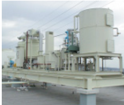
Dichloromethane recovery facility (Ashitaka Factory)
