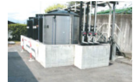
Retaining wall built to prevent leaks of chemical substances (Kofu Factory)
